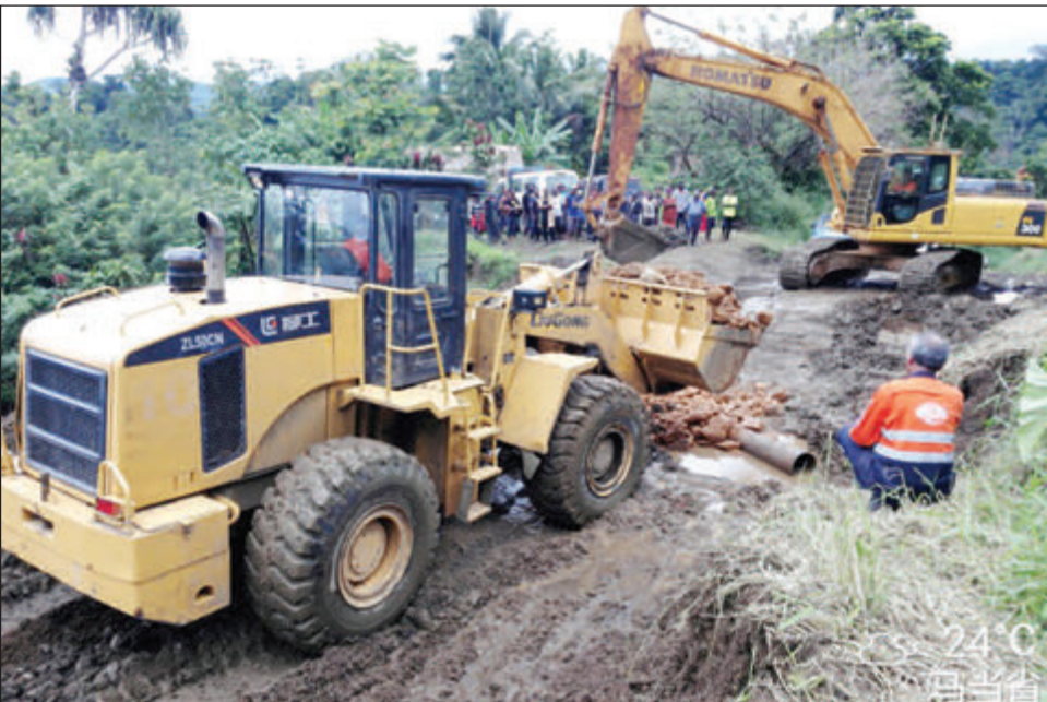
Ramu NiCo-MCC fixed the Iguruwe portion of the road along Madang-Ramu highway during its deteriorating stage
